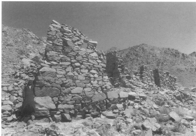
3. The well-preserved, northwest corner of the putative shrine in Wadi Umm Wikala, looking southeast (fig. 10).
